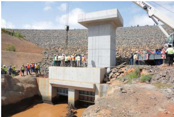
Left. closing of Thiba dam gates.
