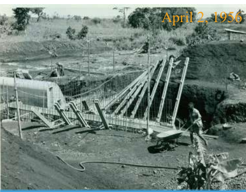
The intake works at Nyamindi River which was to supply water to the Mwea Tebere Irrigation Scheme
